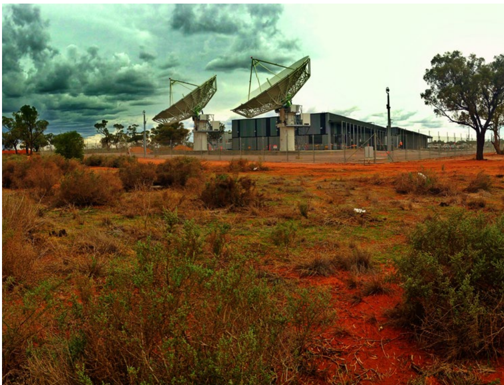
Image: NBN Satellite Ground Station Bourke storm. Credit DITRDCA
