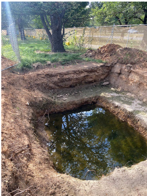
Excavation within TPZ. A review of the roots cut during this dig showed a minimal amount of roots above 20mm diameter were cut. Image credit A. Broman
